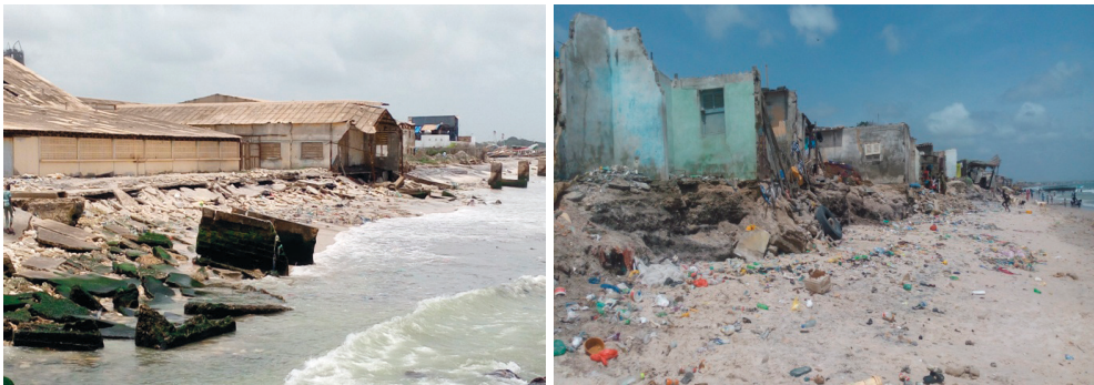
Fig. 13. Ongoing erosion at Rufisque and Bargny Guedj (author's field visit – August 2020)
